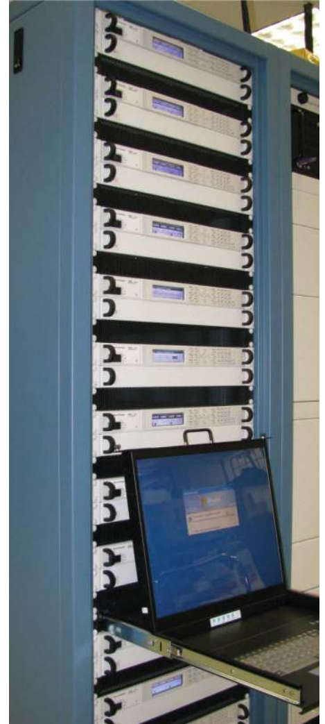
Figure 6. Custom turnkey system
